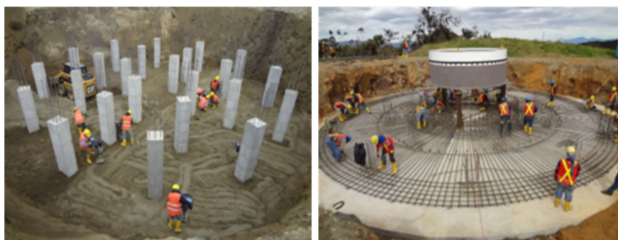
Figure 11. Execution of civil works for the Villonaco wind farm. Courtesy: CELEC EP.
