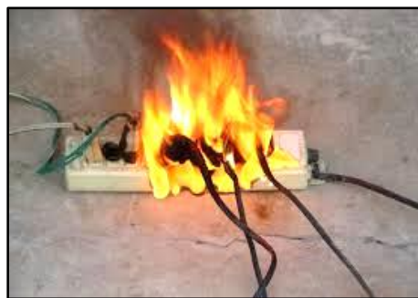
Figure 11. Multiple electricity base catch fire.
