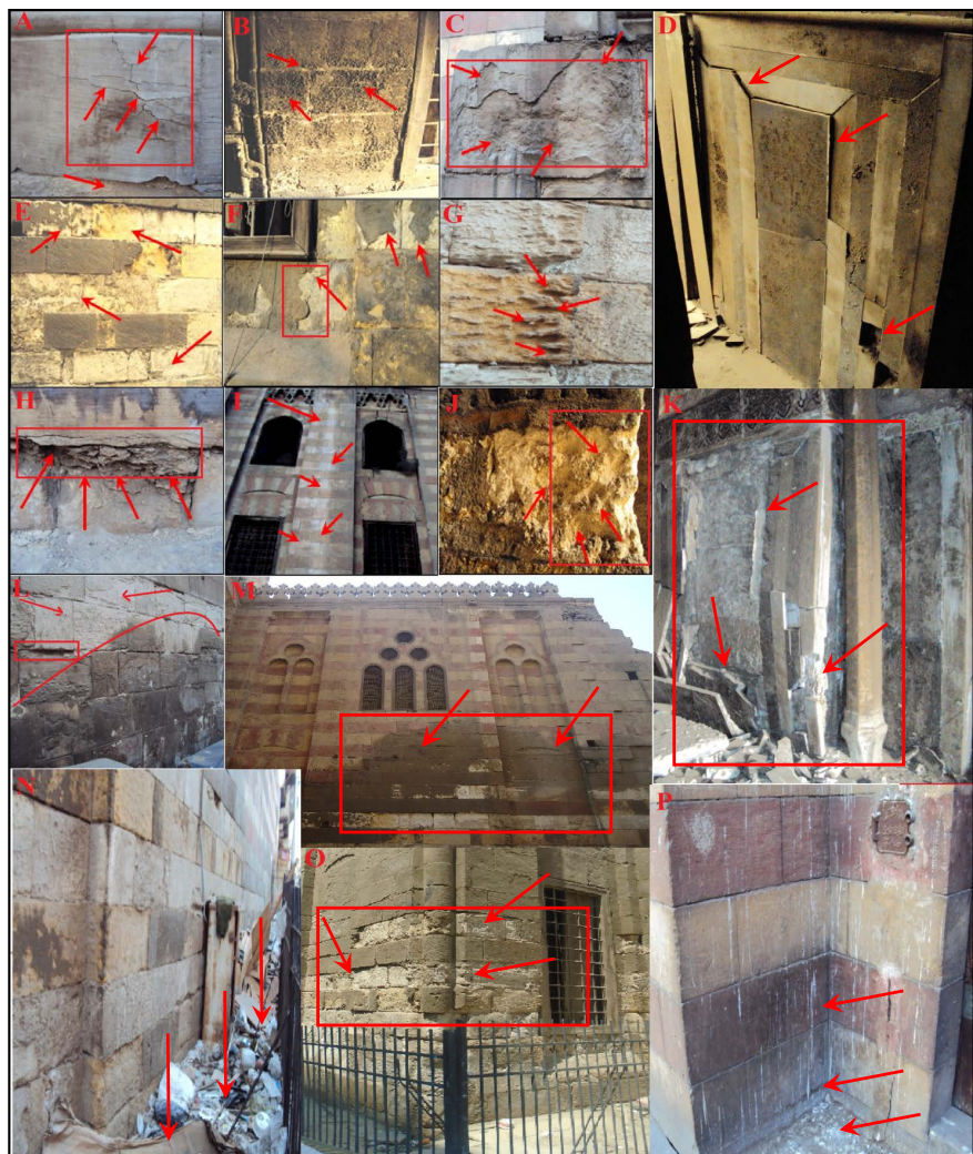
Figure 3. (A, C, E, F, H, I, P) Micro crack, separation to scaling in external layer, Peeling, erosion, loss of stone material of limestone and biological deterioration symptoms (The western south façade). (B) Soiling on the external surface of stone. (G, J, M, N, O) Alveolization, rounding, soiling, erosion, loss of stone material of limestone, and accumulation of rubbish next to the external façade (the eastern south façade). (D, K) Deterioration and fall down of marble casings (the southern wall of the shrine).
