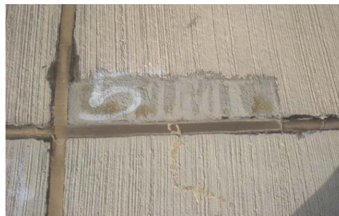
Figure 5. Conceret patch repaired (smaller size) with deformed joint sealant.
