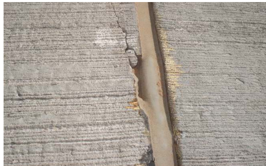
Figure 7. Joint and sealant damage.
