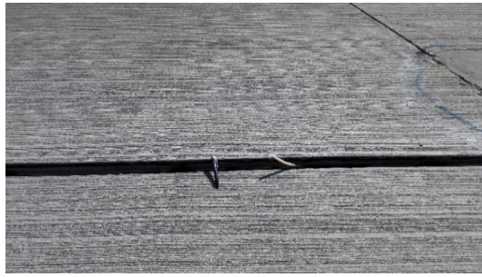
Figure 9. Curling of slabs and poor sealant condition.
