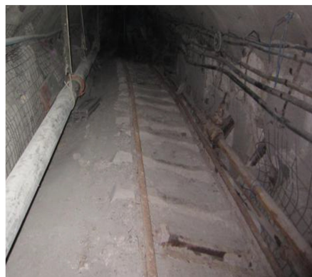
(b) Floor bulging
