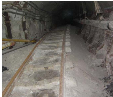
(a) Floor fracture and bulged
