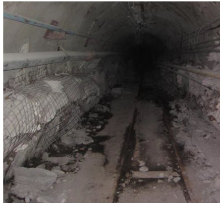
(c) The bottom of the wall is broken
