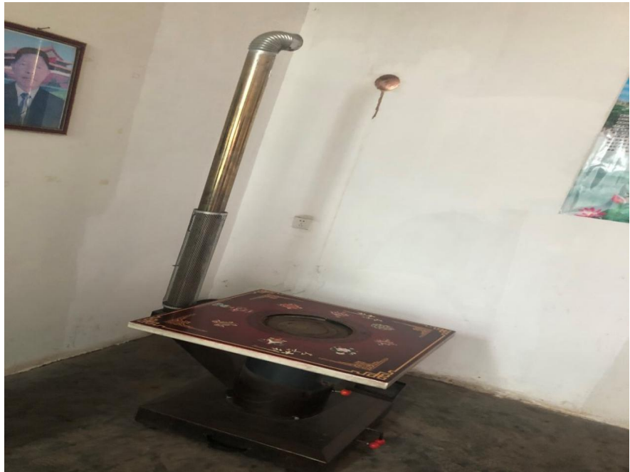
Figure 5. New heating stoves (photo source: author self-photo).
