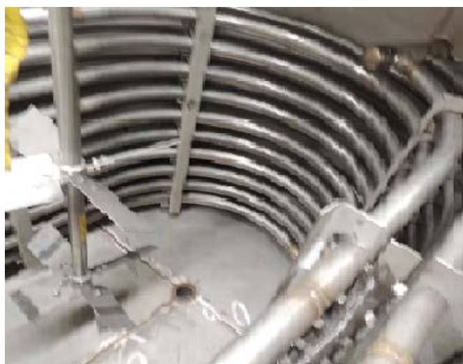
Figure 1. Overview of the shell, coils, and agitators.
