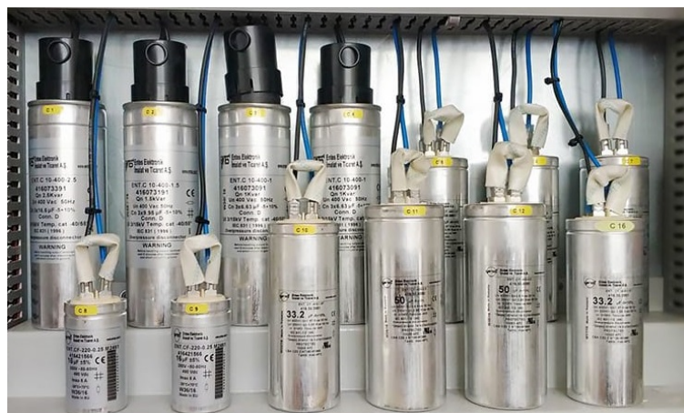
Figure 7. A bank of capacitors for power factor correction [11].
