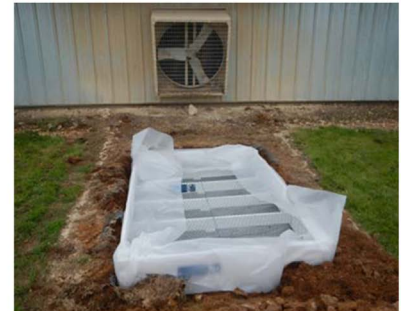
(b) Containment tray with liner
