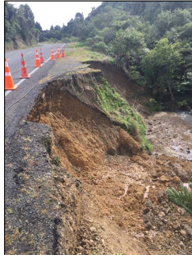
Figure 3. Site 1 under slip (erosion in the base of the road).
