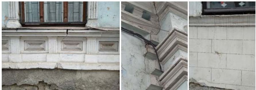
Figure 10. Cracks in walls of architectural monuments. Source: original photos taken by the authors (March 2021).
