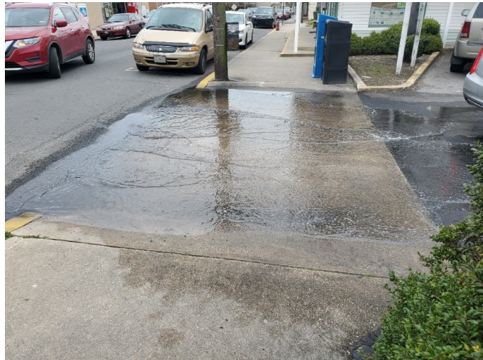
Figure 5. Standing water on sidewalk at curb entrance on main street (Calloway, 2020a).
