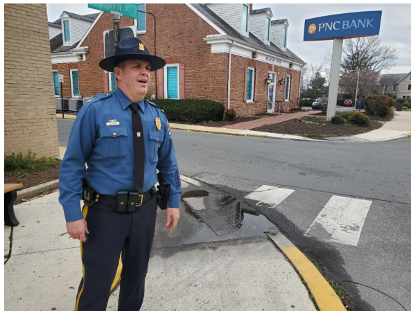
Figure 6. Town of Millsboro police chief standing in front of non-compliant curb ramp on main street (Calloway, 2020b).
