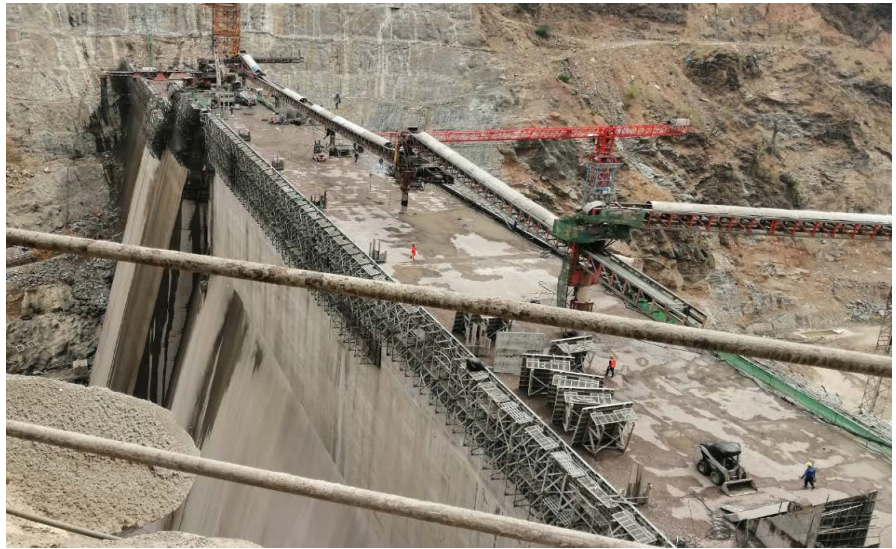
Photo 6. (Upstream) shattered right bank of dam wall.
