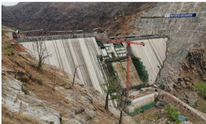
Photo 5. (Downstream) shattered right bank of dam wall.
