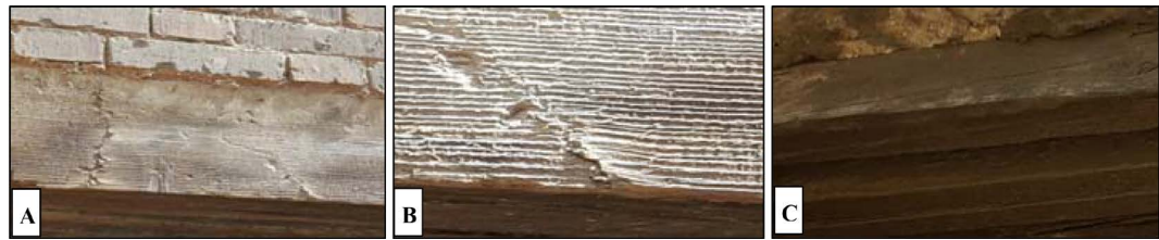
Figure 6. Spread of the different cracks on the pine wood surface, ((A), (B)) the lintel of the door in the mausoleum dome chamber, (C) the window lintel in the outer portico.
