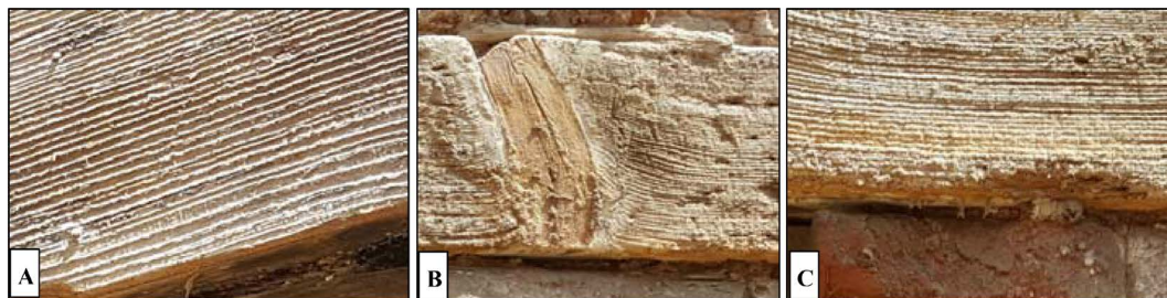
Figure 9. The lintel of the door in the mausoleum dome chamber (A) The roughness of weathered wood surface, (B) the wood knots affected by weathering, (C) the spongy appearance of the wood surface and the erosion of lintel edges.
