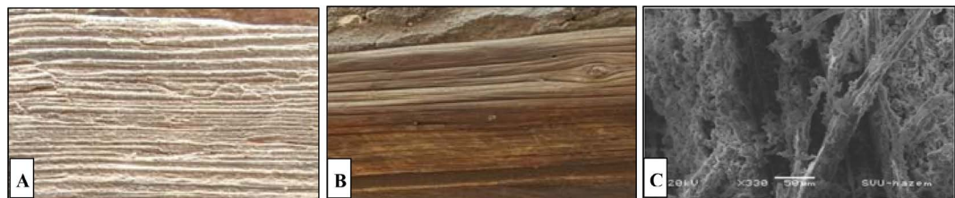
Figure 7. ((A), (B)) The window lintels in the outer portico showing the roughness of weathered wood surface, (C) the accumulated dust particles between the wood fibers, SEM micrograph. 50 \mu m.
