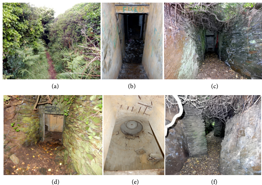
Figure 7. trench—(a) access; (b) R628 (53) entrance; (c) entrance of the 2 nd bunker (61); (d) tobruk (62) access; (e) tobruk weapon room; (f) trench exit corridor.
