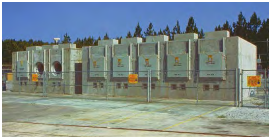
Figure 1. “Dry” storage facility of SNF in the USA.
