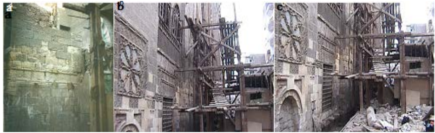
Figure 6. The deterioration aspects at the façade of the Sebil and Kuttab.
