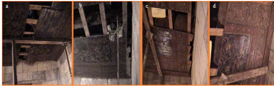
Figure 8. Shows the deterioration aspects of Sebil ceiling before decoding the wooden ceiling units.
