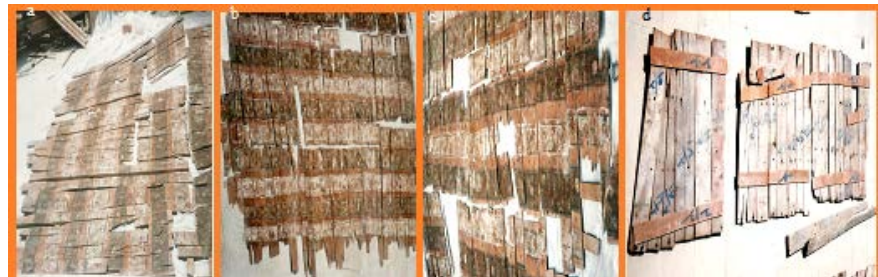
Figure 9. Shows the deterioration aspects of Sebil ceiling after decoding the wooden ceiling units.
