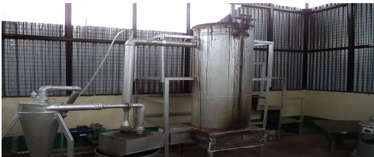
Figure 3. Gasifier in the Shed.
