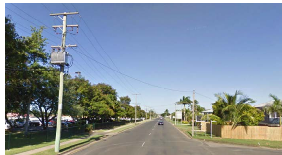
Figure 3. Roadside view of residential load connection from DN.
