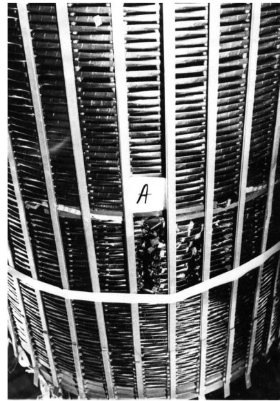
Figure 2. Typical example of deformation due to radial buckling in the A phase LV internal winding of 250 MVA/220 kV transformer ( \Delta X_k = +1\% ).
