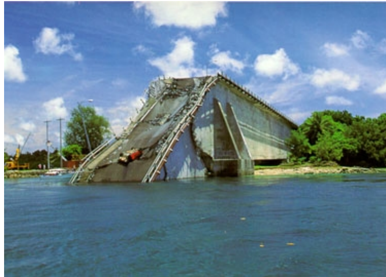
Figure 1. The Koror Bridge collapse.
