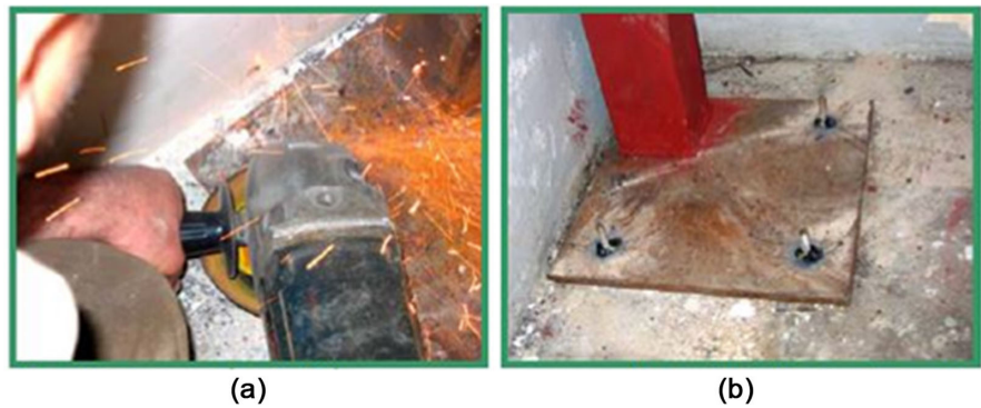
Figure 10. (a) Welding the screws to the column plate and (b) Scouring the upper surface of the screws.
