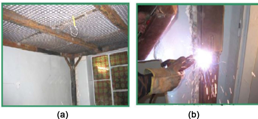
Figure 8. (a) Welding the middle of the column; (b) The final design of the structure after the jacks are released.
