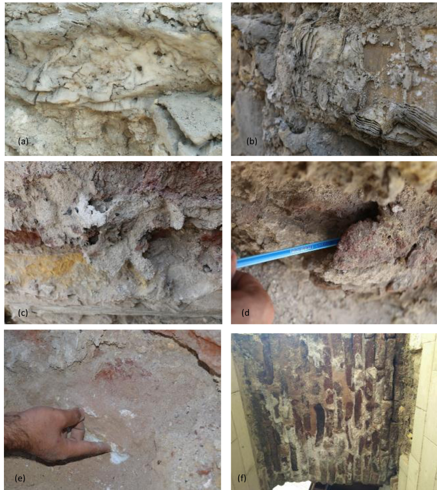
Figure 13. Physical and chemical deterioration forms due to subsurface water rising and salt weathering affecting the roman bricks and structural mortars; (a) and (b) salt efflorescence; (c), (d) and (e) cryptoflorescence, layers exfoliations and hard black crust formation; (f) brick and joining mortars disintegration due to salt weathering mechanisms.
