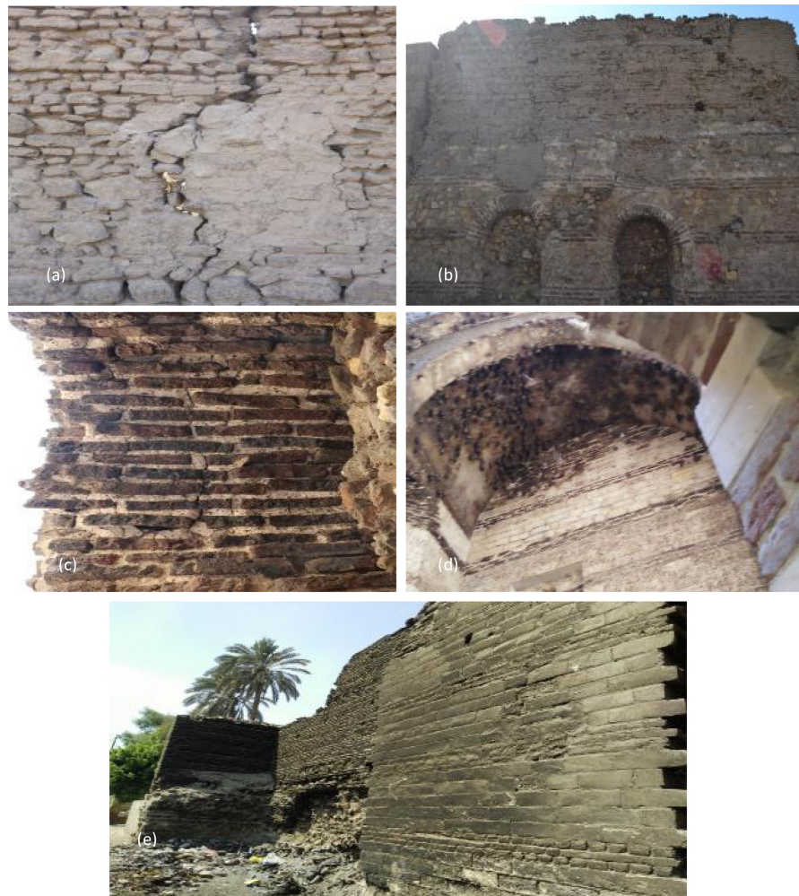
Figure 12. Structural deficiency of many walls and towers of the Babylon of Egypt: (a) cracks and fissures in the vertical walls; (b) permanent deformation of the bricks in the zone of the borders and main wall of the façades; (c) danger cracks appeared in some towers; (d) one very significant source of surface damage resulted from the fesses of bats that inhabited the tower in thousands. And (e) separation between the façade and the radial walls are obvious.
