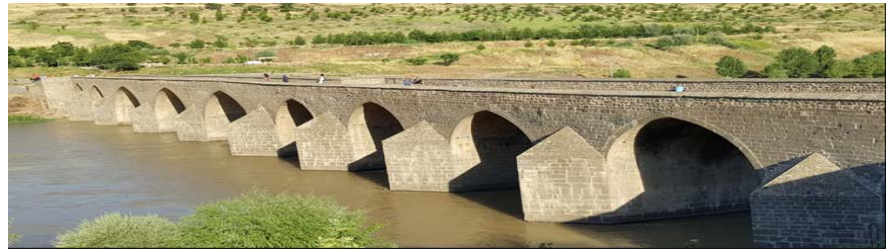
Figure 2. Capped pyramidal flood splitters on the upstream face.
