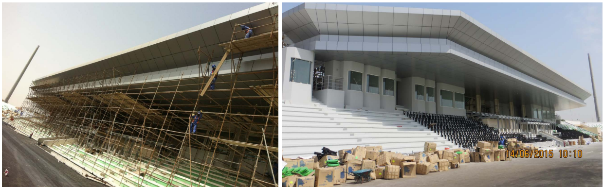
Figure 2. View of the canopy after the cladding work (left) and after the installation) (right).
