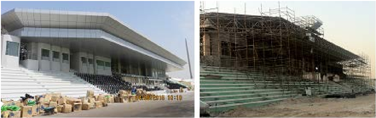
Figure 1. Views of the cladding work (left) after finishing of the cladding and (right) during the execution.
