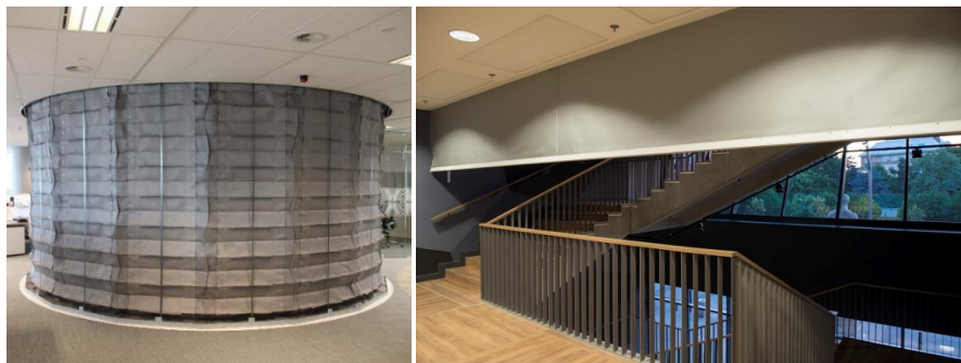
Figure 12. Separation of exit routes by fireproof curtain in a building (Courtesy of Greene Fire [62]).
