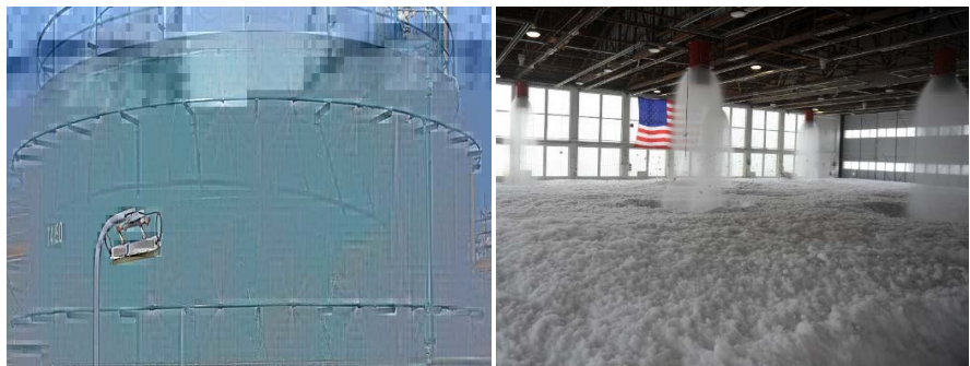
Figure 6. Deluge fire sprinkler system with water and foam (Courtesy of AusIMM – The Minerals Institute [49]).
