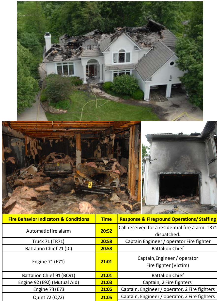
Figure 2. Effect of fire on a residential building without fire sprinkler system (Courtesy of the National Institute for Occupational Safety and Health (NIOSH) [20]).
