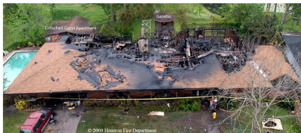
Figure 1. Example fire damage to a residential building (Courtesy of NIST Technical Note 1729; http://ws680.nist.gov/publication/get_pdf.cfm?pub_id=909779 ).
