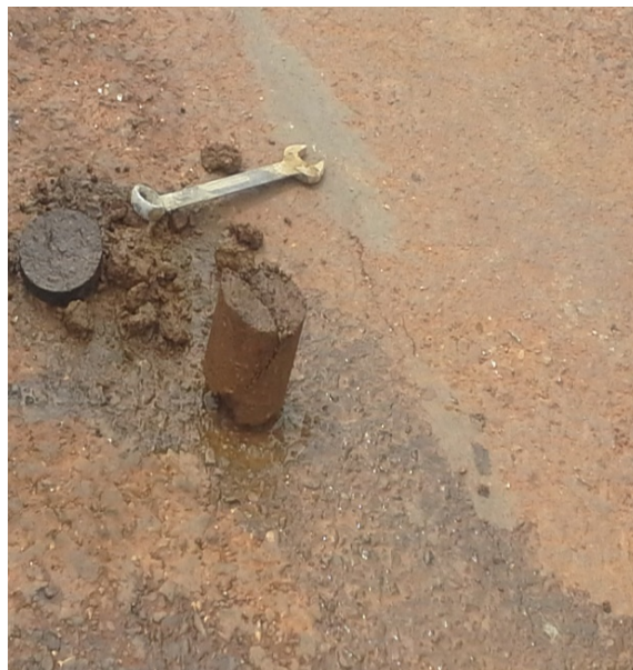
Figure 1. Core extracted from cracked section on the road.
