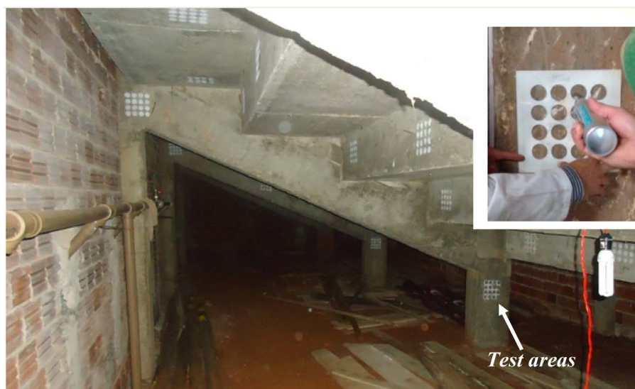
Figure 4. Indication of the hardness test areas on the exposed concrete surfaces of the structural elements under the bleachers (insert scelerometer).
