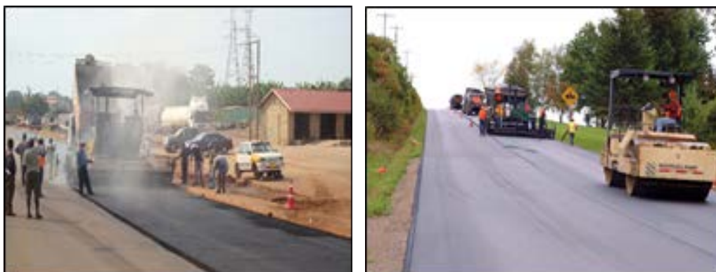
Figure 1. Fumes from HMA (left) and none from WMA (Right) [Photo: Croteau and Tessier [17]].
