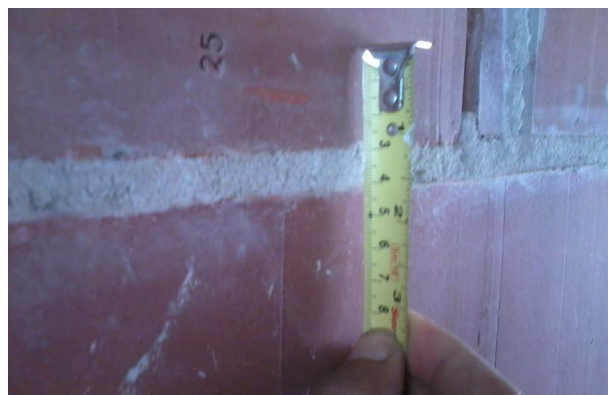
Figure 2. Joints within specifications.
