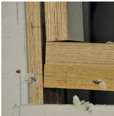
Figure 22. Falling down of Panel-B from LVL frame. opening (SWWOS).
