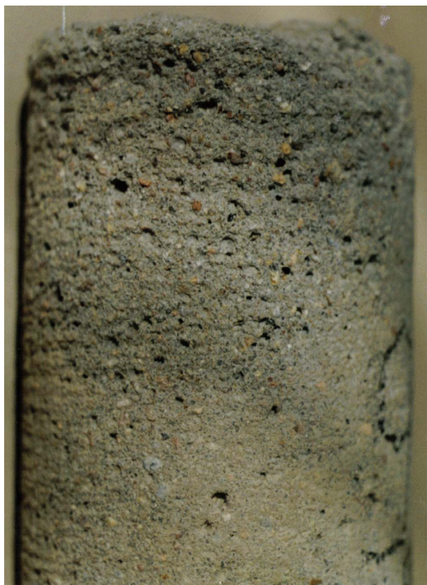
Figure 5. Top layer of floor is most porous and weakest.
