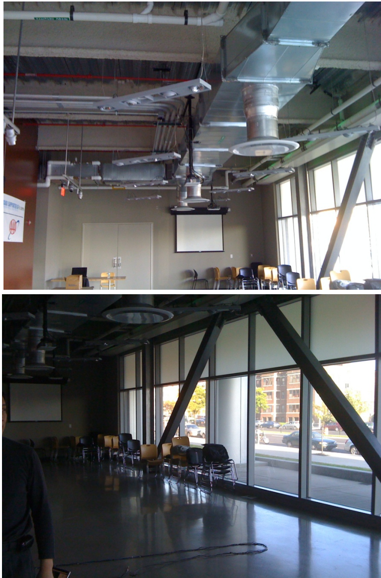
Figure 4. Noise sources in the room under test including the street, and the air conditioning unit.
