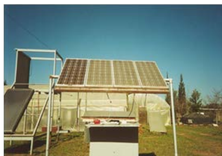
Figure 2. Four solar panels.
