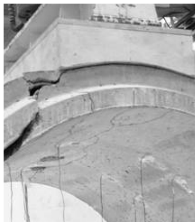
Figure 13. Rupture of a test piece under vertical loading.
