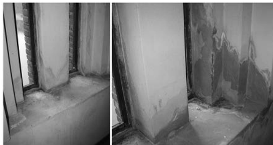
Figure 10. Observed moisture spots at the inner surface near the windows.
