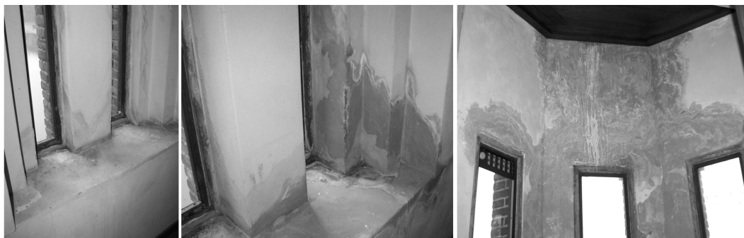
Figure 2. Observed moisture damage in the tower of the building: moist spots and efflorescence.
