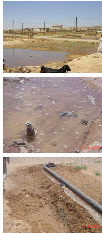
Figure 7. Examples of technical losses: left-broken pipe; middle-leaking pipe; right-breaking pipe to supply water to livestock.
