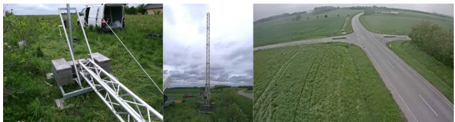
Figure 16. The TRG-pole is deployed at a traffic intersection with limited existing infrastructure.
