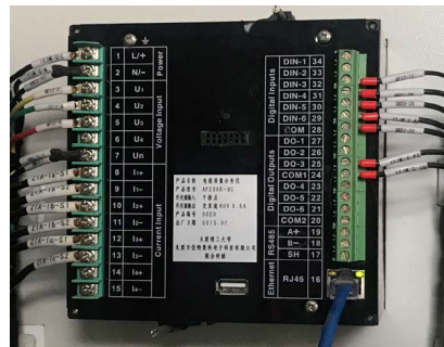
Figure 1. Power monitoring module (AP2008-9C).
