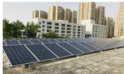
Figure 3. Outdoor PV module performance testing setup at taiyuan university of technology, China.
