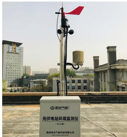
Figure 2. Photovoltaic power station environment monitoring setup (PC 6).
