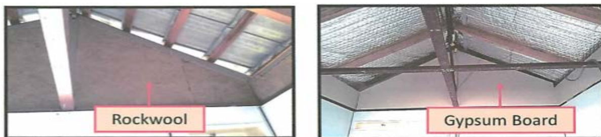
Figure 2. Radiant barrier systems between the ceiling and roof of a building enclosure.
