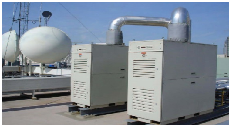
Figure 2. Natural gas based micro turbine units (65 kW × 2) at Goldwind Co. Ltd.
