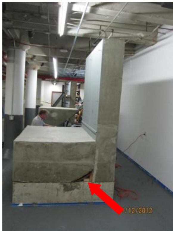
Figure 7. The PWR basemat mockup, “G”, following placement of concrete. Red arrow points to curved region of the liner.
