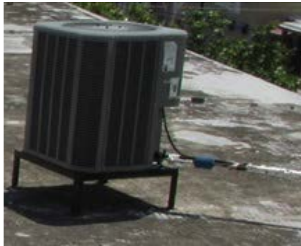
Figure 7. Fan-coil type AC unit with incomplete lining. Source: Own elaboration.
