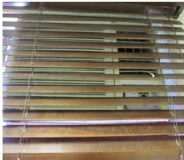
Figure 5. Window type AC unit with air outlet obstruction. Source: Own elaboration.
