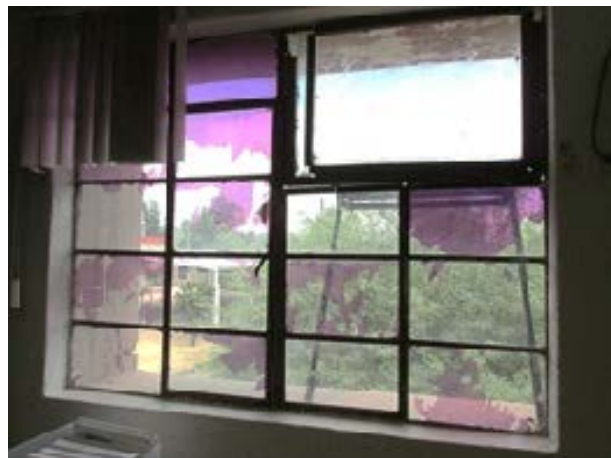
Figure 2. Blacksmith-structured window with damaged polarizer film. Source: Own elaboration.
