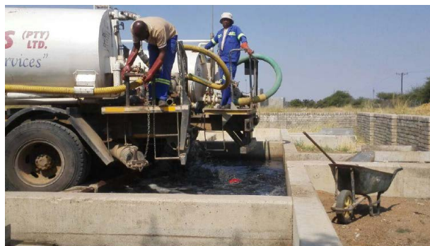
Figure 5. Example private vacuum track discharging at the Gaborone wastewater treatment plant (GWWTP) discharge bay.
