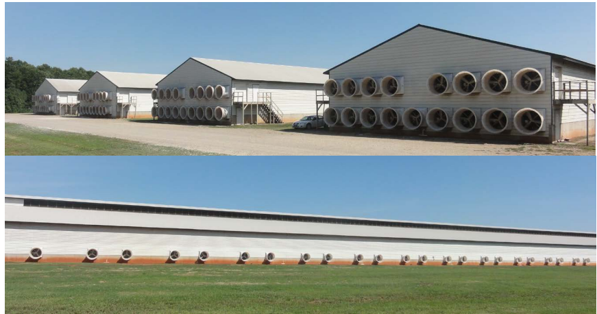
Figure 3. Illustration of the fans in tunnel-ventilated houses (top) & a cross-ventilated house (bottom).
