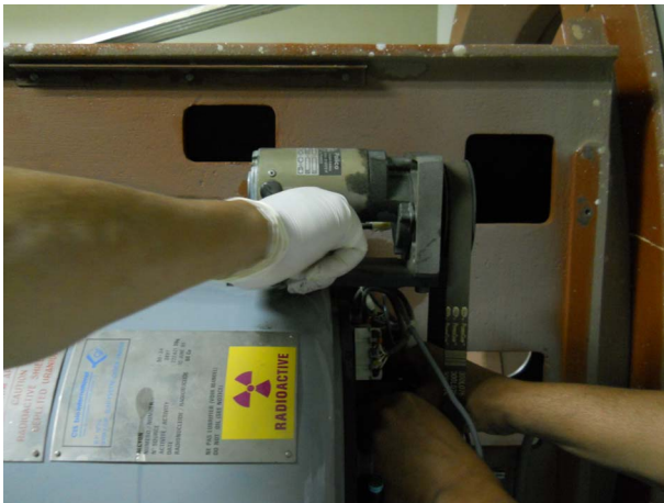
Figure 6. Disconnection of power source wire.
