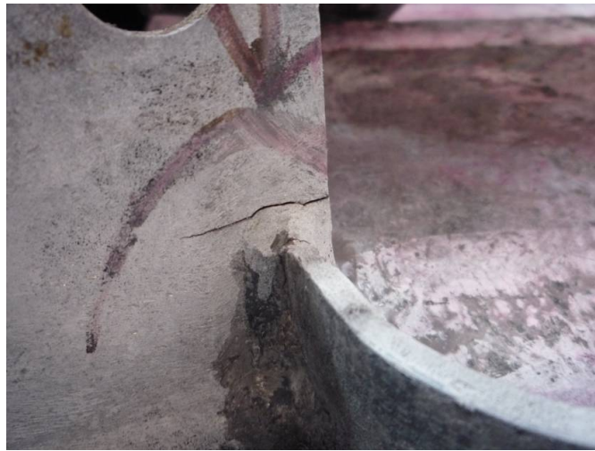
Figure 2. Crack on the nozzle bracket.
