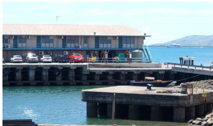
Figure 4. The tide-gauge station is located at the main wharf of Lautoka consisting of heavy construction resting on soft marine sediments. The load is bound to generate site-specific subsidence, seriously affecting the tide-gauge record.
