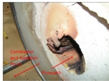
Figure 2. Image of large deposit formation on the left size of the transition piece [12].
