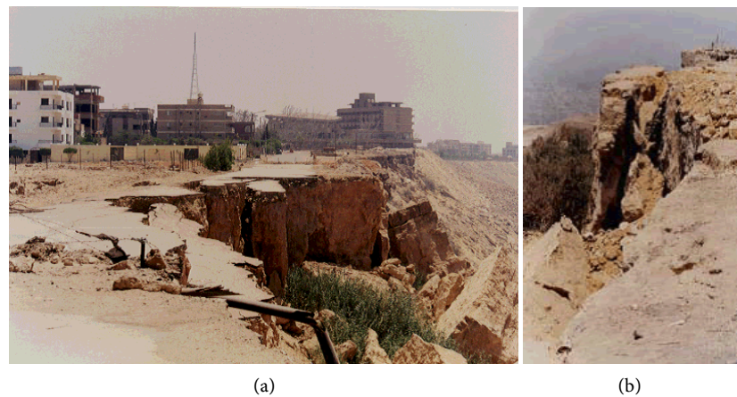
Figure 2. (a) Urban communities close to the steep cliffs of the Southern Upper Plateau; (b) rock cracks and failure along the cliff.
